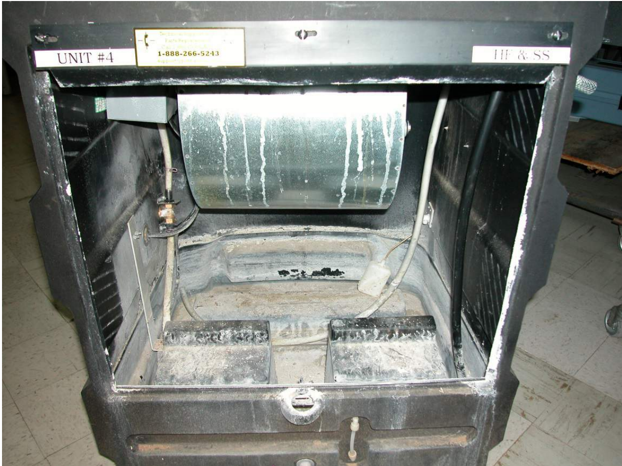
Figure 14. Post-test images of scale and sediment in Unit #4 (SS/HF)
