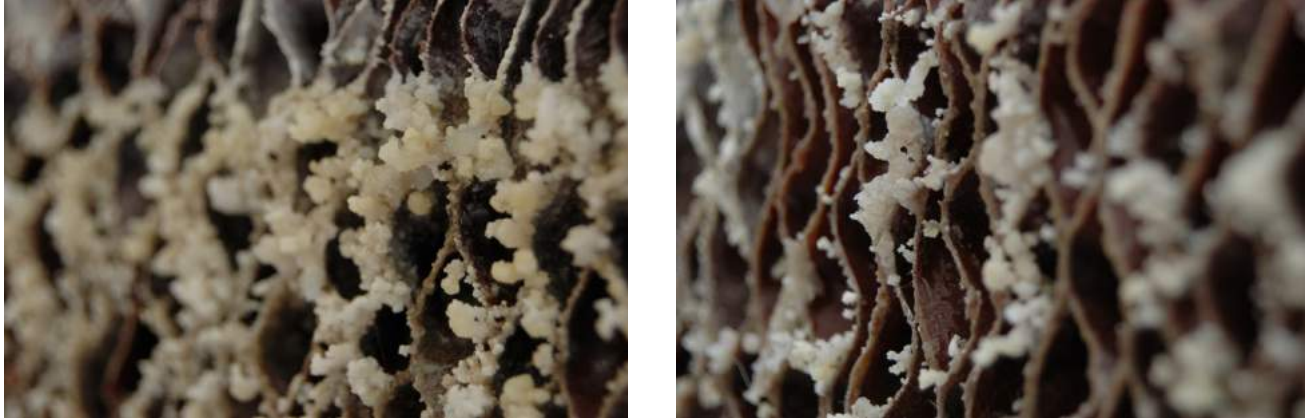
Figure 13 a and b. Post-test images of scale build up on the evaporative cooler pads. a) left - Side-stream filter only Unit #2 and b) right - Control Unit #1
